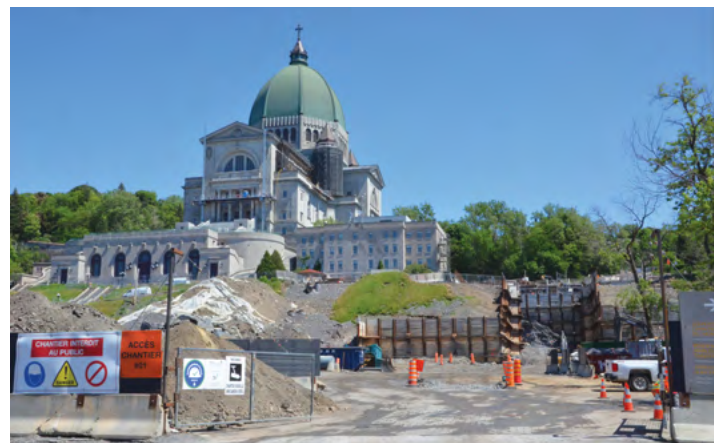
A vast construction site gives a glimpse of the location of the future building, which will be accessible as soon as you enter the site. Photo: André Charron, CSC
